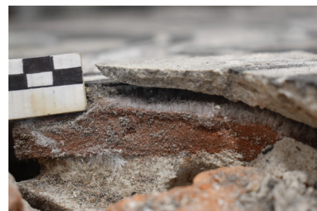
Picture 3. Detail of nitromagnesite salt efflorescence developing between the bricks and the surface.
