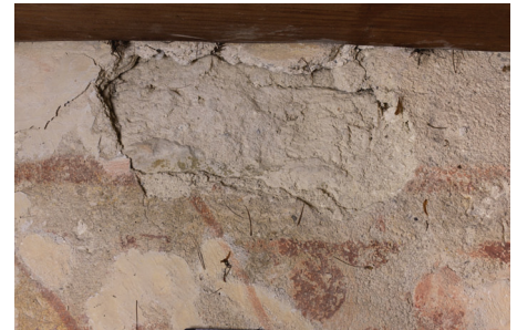
Picture 3. North wall of the nave, detail of the wall painting next to St. Christopher showing plaster losses, delamination and the heterogeneous surface, SUPSI, 2025.
